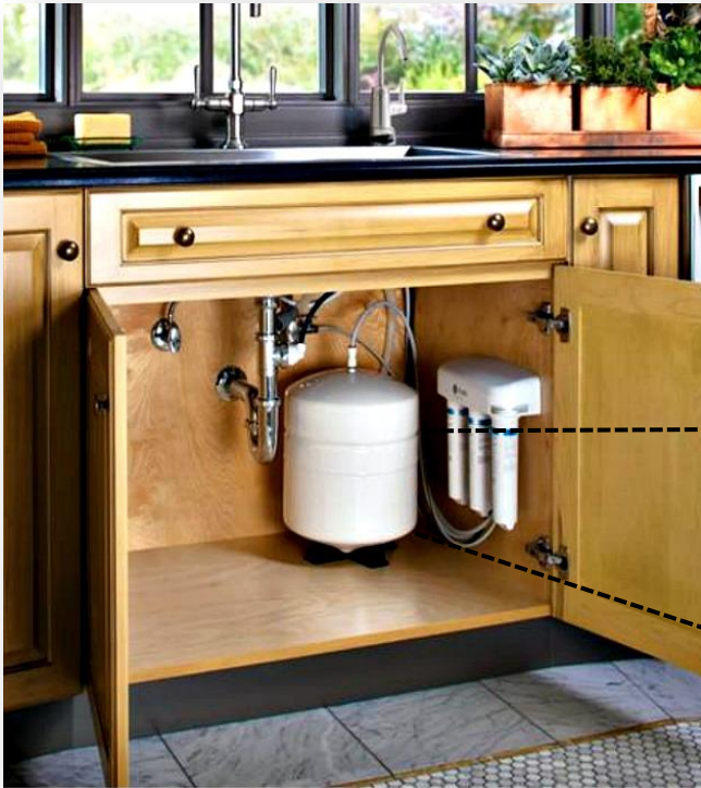
Exhibit 2: Reverse Osmosis and 3-Stage UTC water filtration equipment
